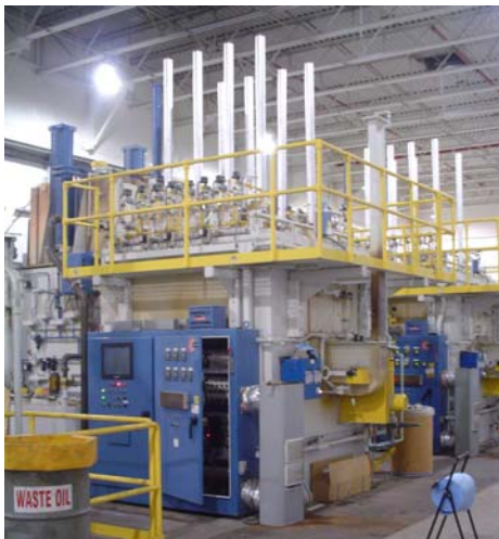
SEW-Eurodrive's heat transfer system was installed by GreenWood along with all equipment for the facility expansion completed in 2005
